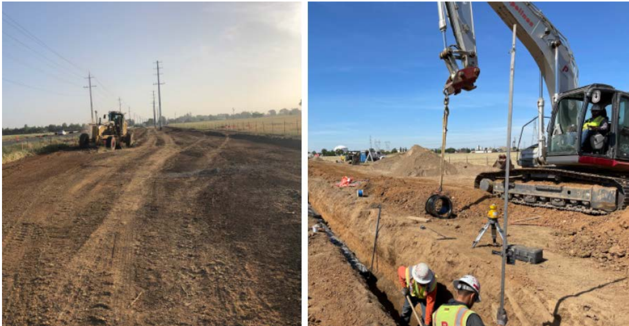
Pictures 2 and 3 – Roadway Excavation east of Grant Line Rd and intallatoin of 16-inch water line
